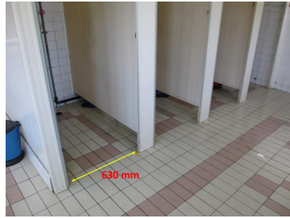
Figure 5.2.52: The narrow bathroom without sufficient space.
