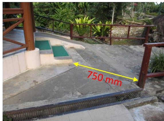
Figure 5.2.50: The condition outside the changing room and toilet.
