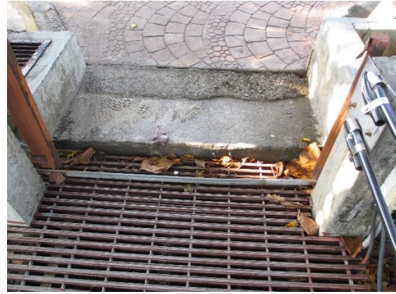
Figure 5.2.8: The small step at the pier entrance
