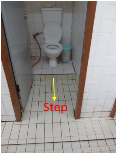
Figure 5.2.53: The inaccessible toilet.
