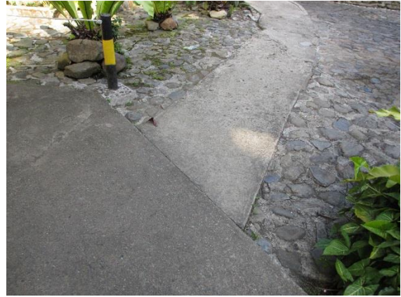
Figure 5.2.40: The uneven and small width path
