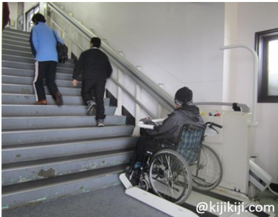
Figure 5.2.57: The wheelchair platform stairlift in the station
